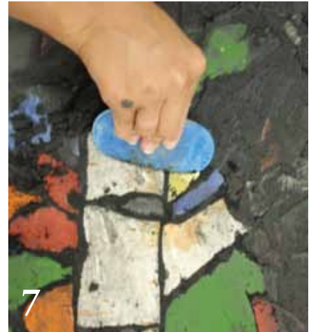
7 Scrape away all the grout that's not in the gaps between the tiles.
