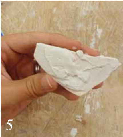
5 Smooth the glue to a thickness of 1/8 inch on the back of each tile.
